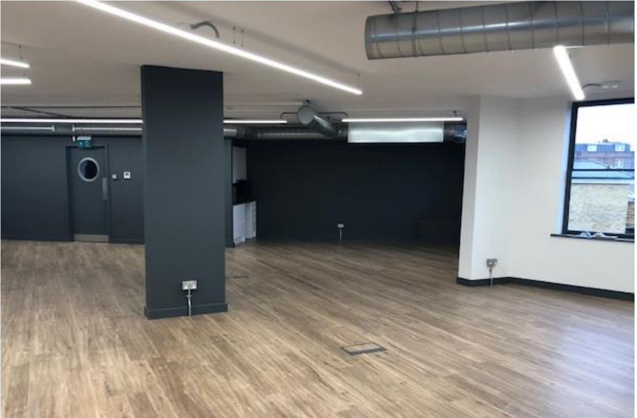
Third Floor with floor boxes
